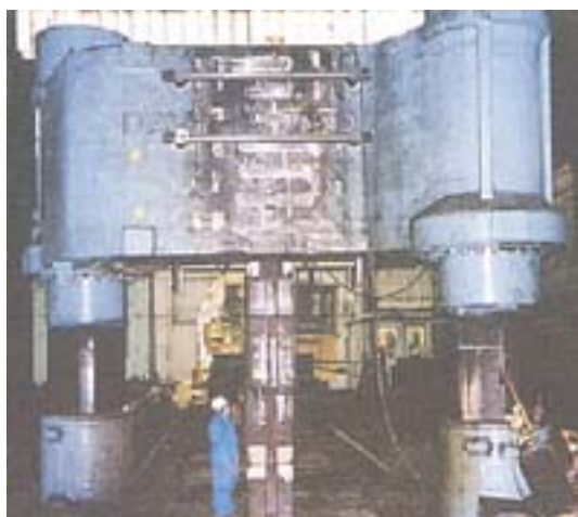
The Metallock repair was enhanced by fitting tie rods. The repair was so good that the new crosshead was never used
