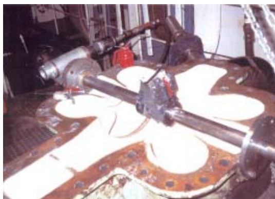
The Metallock repair, carried out offshore, involved the application of a flake glass coating material followed by machining using line boring techniques to recut wear ring glands.
