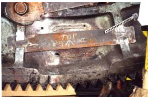
The 6.5 metre diameter cast steel gear developed cracks emanating from four of the oval windows between spokes. As well as metal stitching plates into the windows, Metallock stitched tie plates across the ovals to provide extra strength
