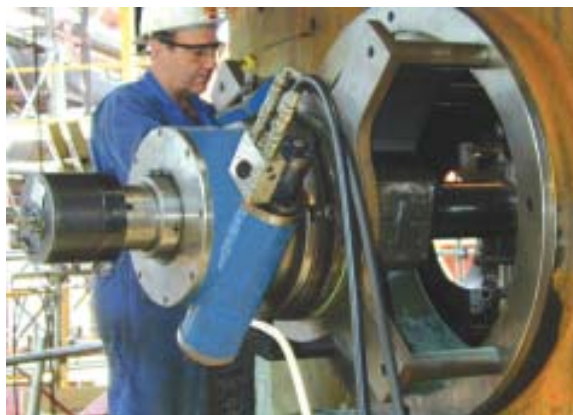
Two Metallock purpose-designed boring machines were used simultaneously to speed up the boring of 15 hearth shell bores to accommodate tapered tuyere cooler holders at Dofasco Inc, Canada.
