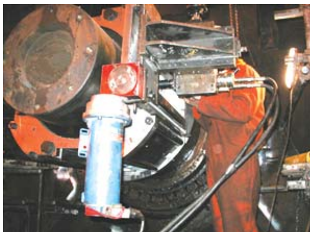
The in-situ machining was very accurate and better than machining the hub in a workshop.
