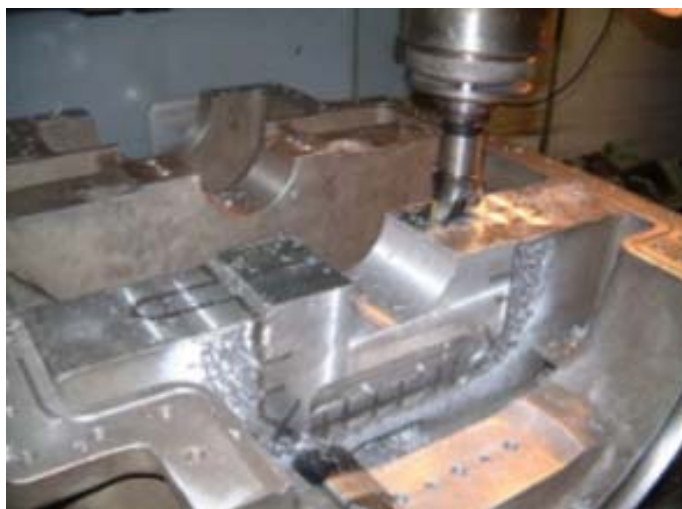
On completion of the Metallock repair, the bore, journal pocket sidewall and joint face were machined to the customer's specification.
