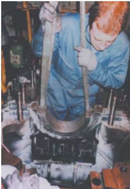
To effect the repair, the damaged pocket was cut out by chain drilling, machining and hand fitting, to accept a steel insert machined from a single solid piece of steel to precisely fit the shape formed in the bedplate.
